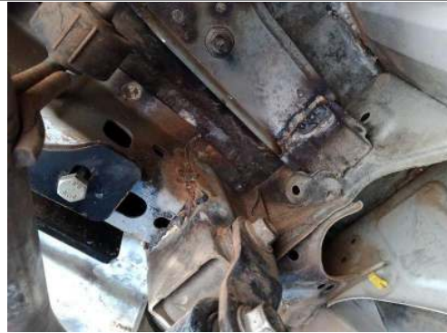
Main Beam Right
