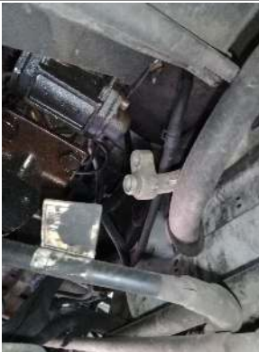
Air conditioner pipes
