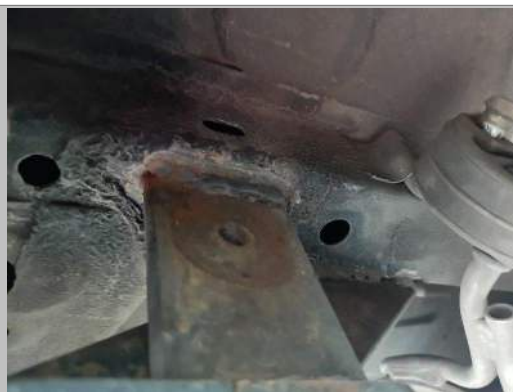
Main Beam Right
