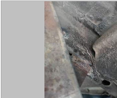
Main Beam Right
