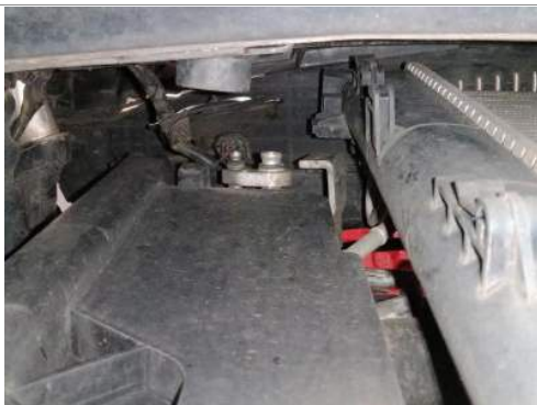
Air conditioner pipes
