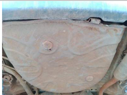
Inner Boot Floor Pan and Spare Wheel Well
