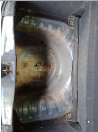
Inner Boot Floor Pan and Spare Wheel Well
