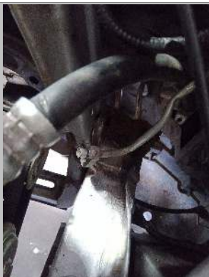
Air conditioner pipes
