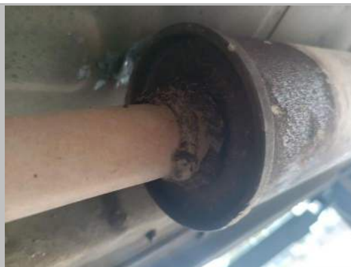
Engine to silencer pipe
