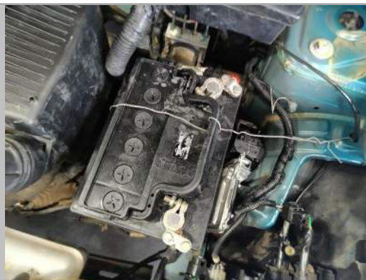
Battery is loose
