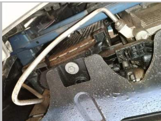
Air conditioner pipes
