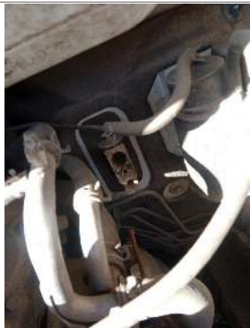
Air conditioner pipes
