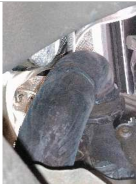
Engine to silencer pipe
