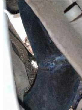
Engine to silencer pipe
